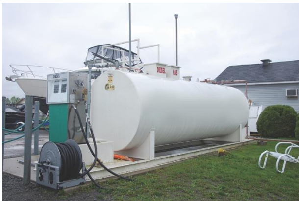
Storage of liquid fuel
