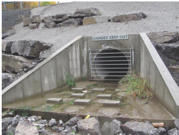
Stormwater discharge outlet
